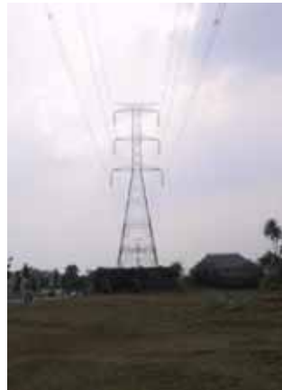
A high transmission cable stretch out above the site ground. (photo by Adi Purnomo)
