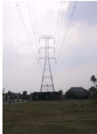
A high transmission cable stretch out above the site ground. (photo by Adi Purnomo)
